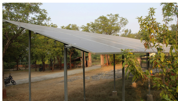
Solar Electricity Panels
